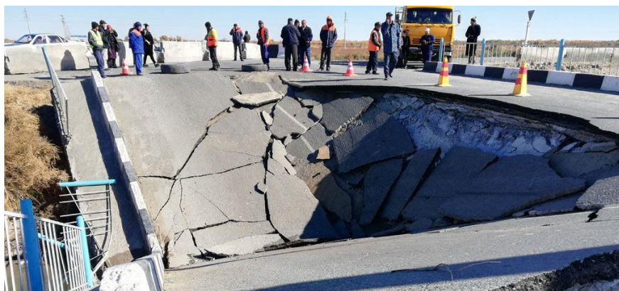
Figure 2. The base of the bridge located on the 16-21 km section of the 3rd category 4R35 “Jizzakh (4R38 automobile road) -Pakhtakor-Dustlik-Gagarin-M39 automobile road (128 km)” automobile road of Pakhtakor district damage to the structure as a result of salinization of soils
